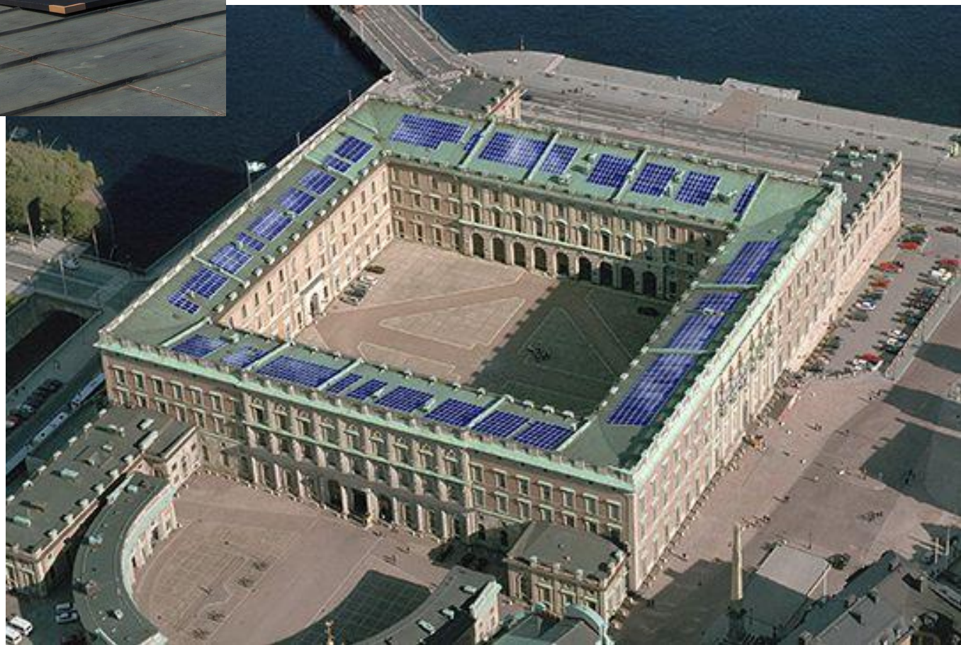
The King of Sweden helping to place solar panels on the roof of the Royal Palace of Stockholm (Sweden)
