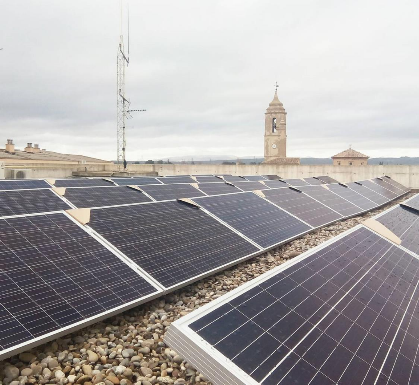
Solar panels on a flat roof with parapets (Spain)
